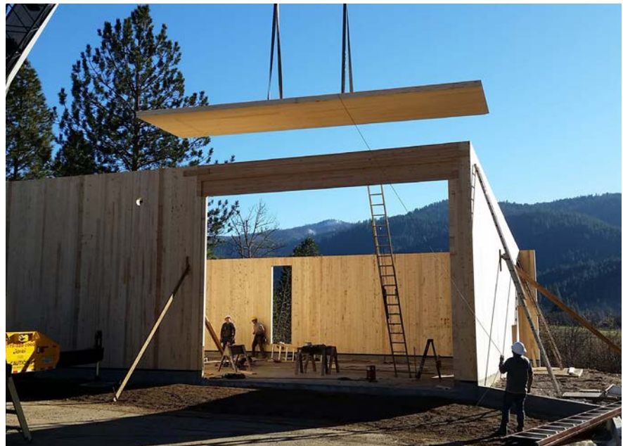
CLT wall and roof panel being hoisted into place at California's first all CLT building in Quincy, CA
